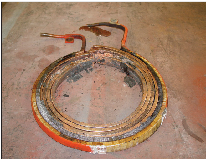
Figure 3. Multi-layer coil failure.
